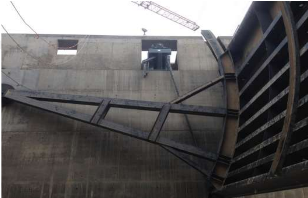
Figure 3.9: Radial Gates and Its Lifting Mechanism ( www.vortexhydradams.com )
