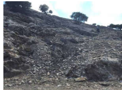
Figure 10. İmambaba Peak road location, highly fractured Permian marbles.
