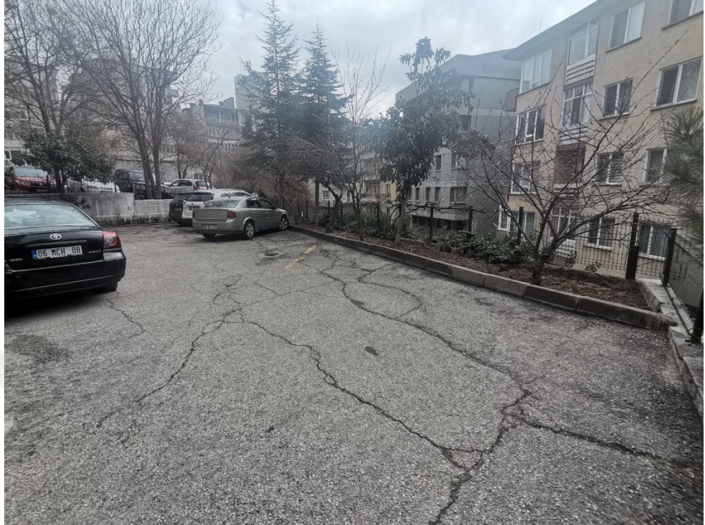
Figure 63. Existing condition of Patch 63.
