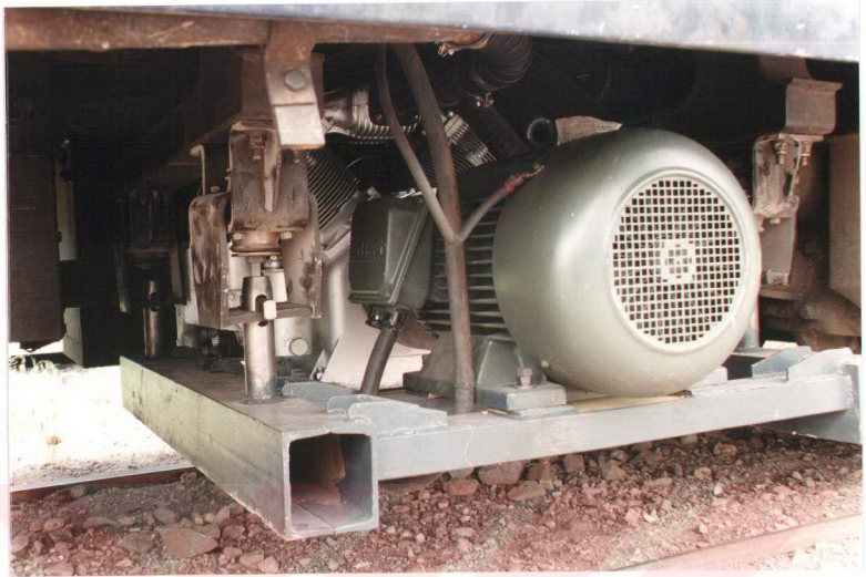
Fig. 33 Photograph of the compressor motor with the compressor
