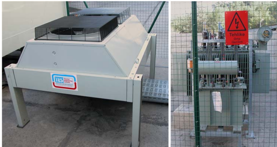
Figure 3.19 HX Unit and Coupling Transformer
