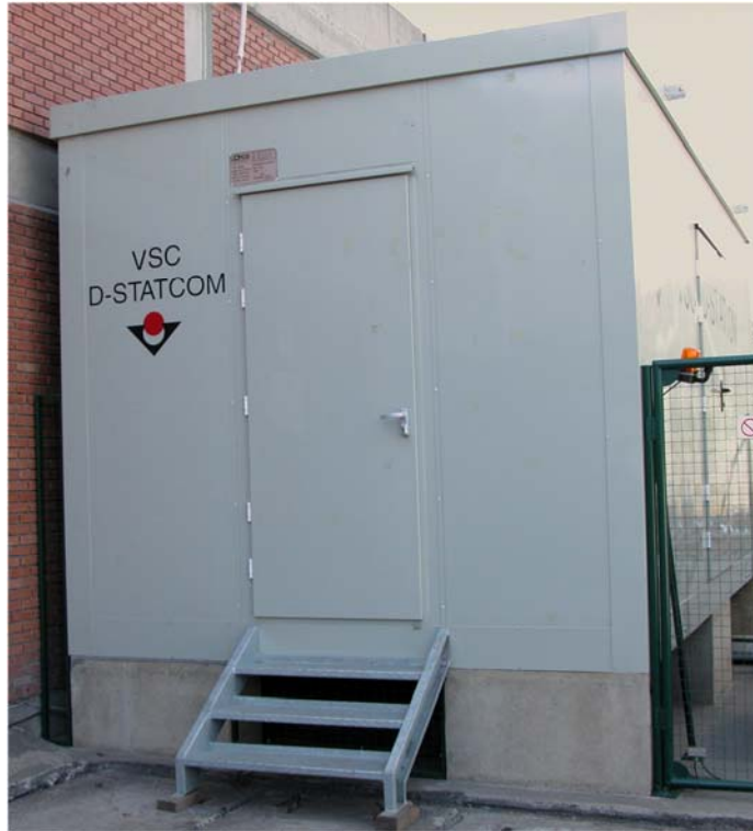
Figure 3.18 STATCOM LV Container
