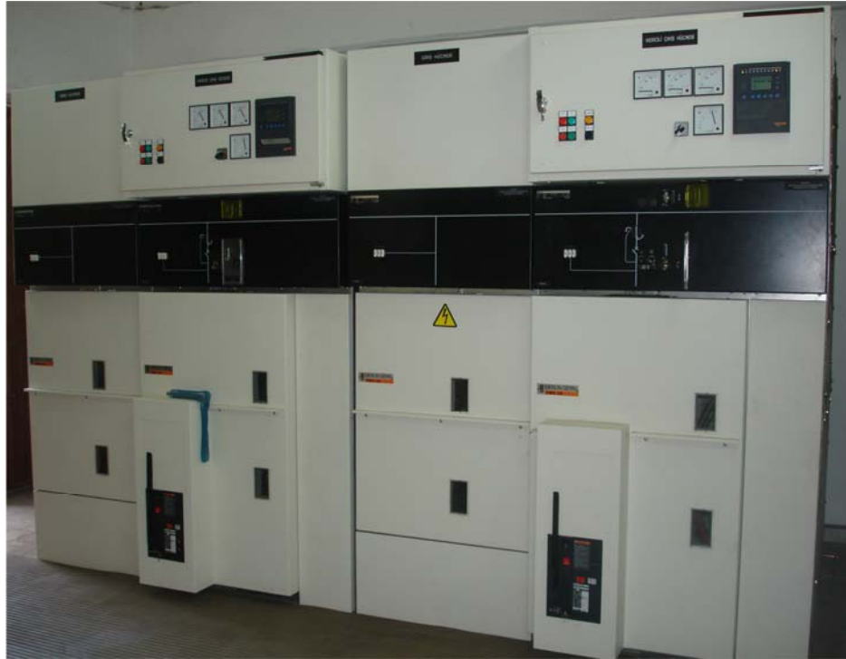
Figure 3.17 6.3kV Switchgear Cubicles
