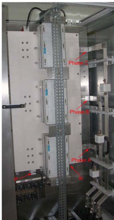
Figure 4.4 Implemented Power Stage of VSC
