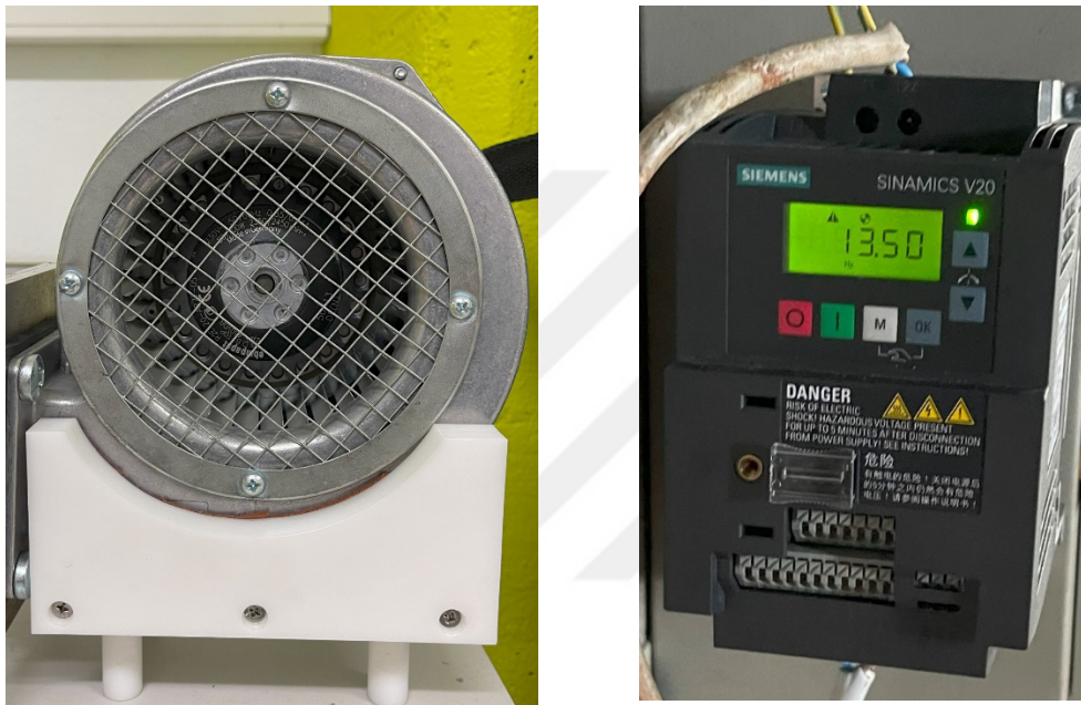
Figure 2.8 The fan and inverter device
